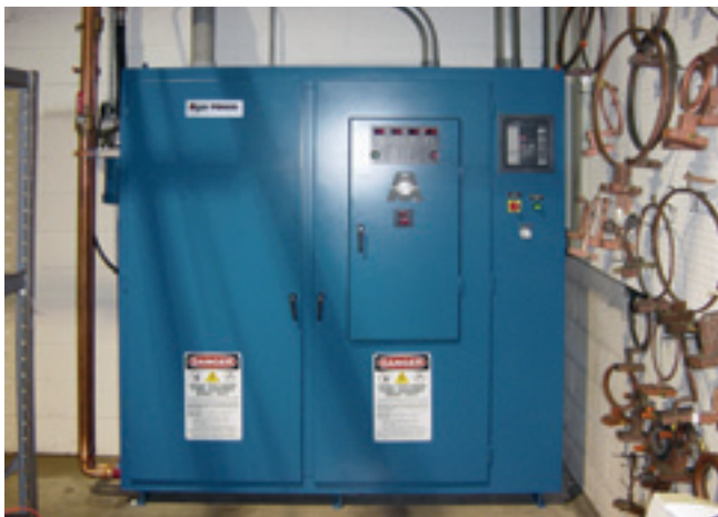
Fig. 2 Most recently installed 250 kw, 4-10 kHz power supply
